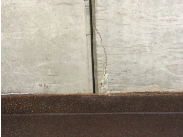
Minor damage noted to panel 3 at left bank
