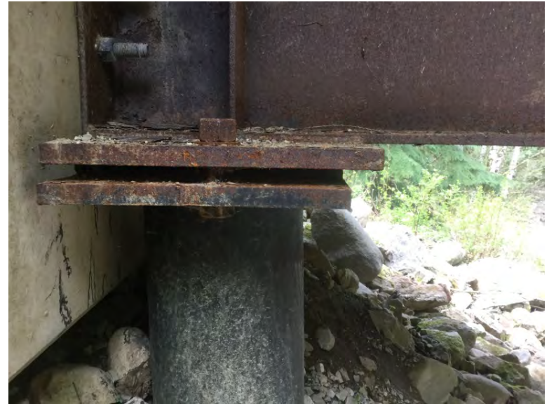
Bearing plates misaligned at upstream left bank
