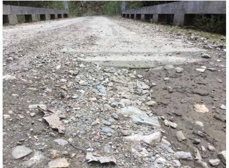
Ballast wall at left bank is 30mm lower than deck panel
