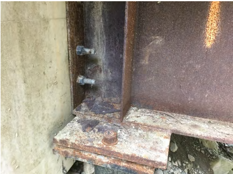
Minor steel delamination
