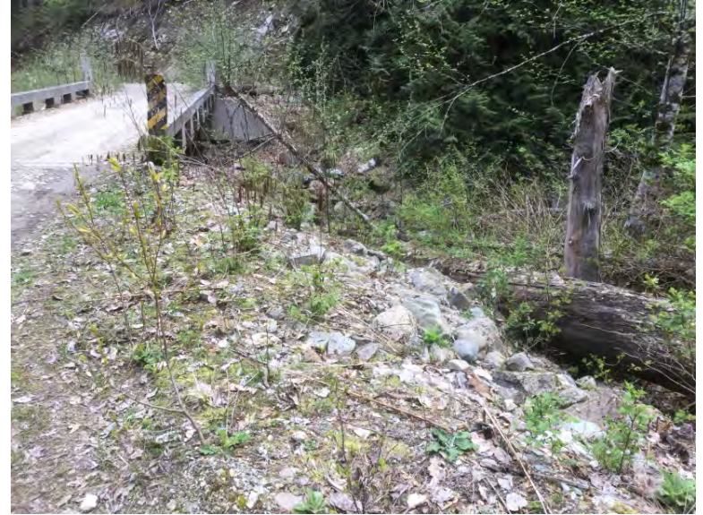
Missing upstream left bank fender, has rolled off road
